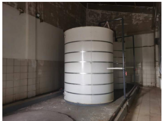
串湖污水厂次氯酸钠加药桶
